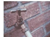
Shut off water supply to hose bibs
