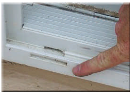
Exterior window weep holes must be periodically cleaned
